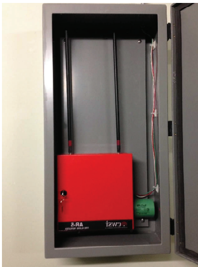
AR-5 Repeater Installed in ES321606-FR2 Enclosure
